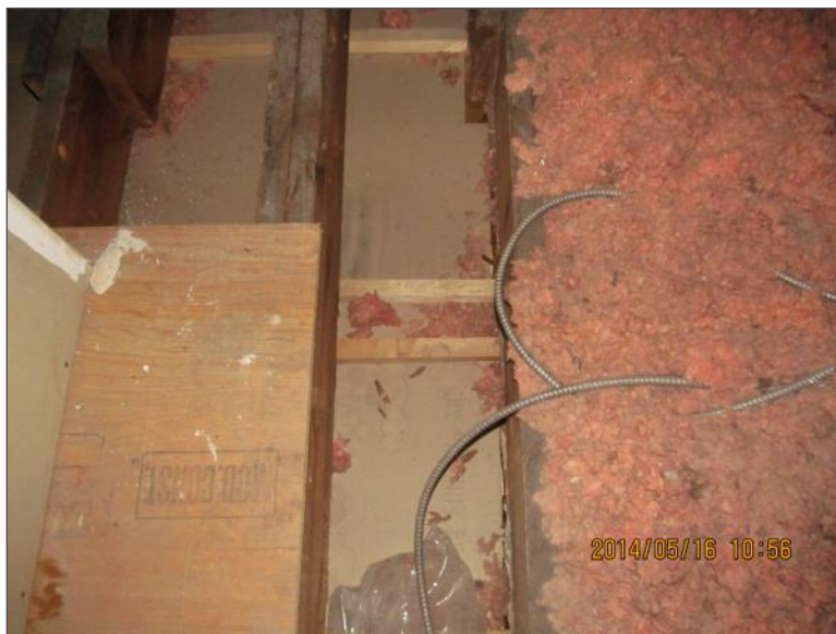
Example of attic insulation not providing full coverage of the second floor ceiling.
