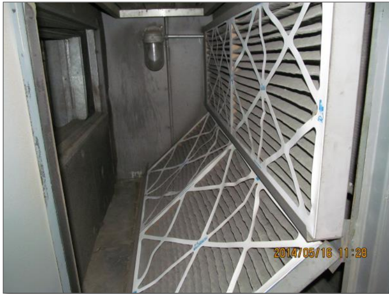
Example of dirty air filters in the AHUs.
