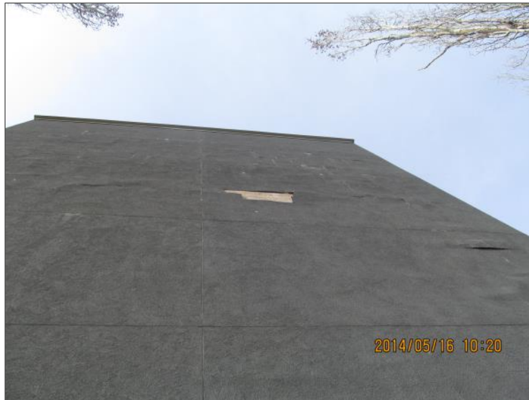
Example of the exterior coating on the Durisol Block wall failing.
